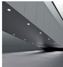
Soffit LED spot cladding lighting
